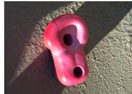
Ross' Landing Park: Replacement wall climber pegs were identified as needed on multiple occasions.
