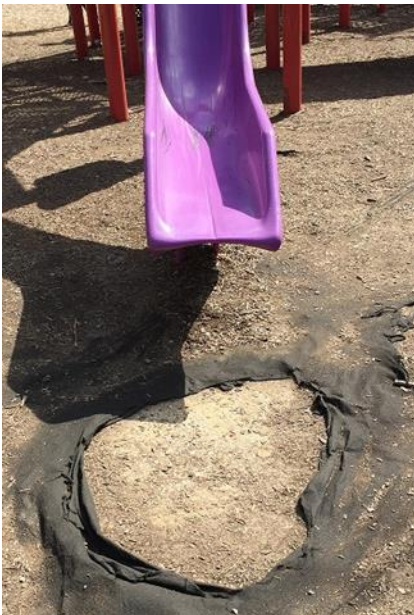
East Lake Park: Drainage issues continue to strip the playground of mulch. The inspector identified the safety hazard on numerous occasions.
