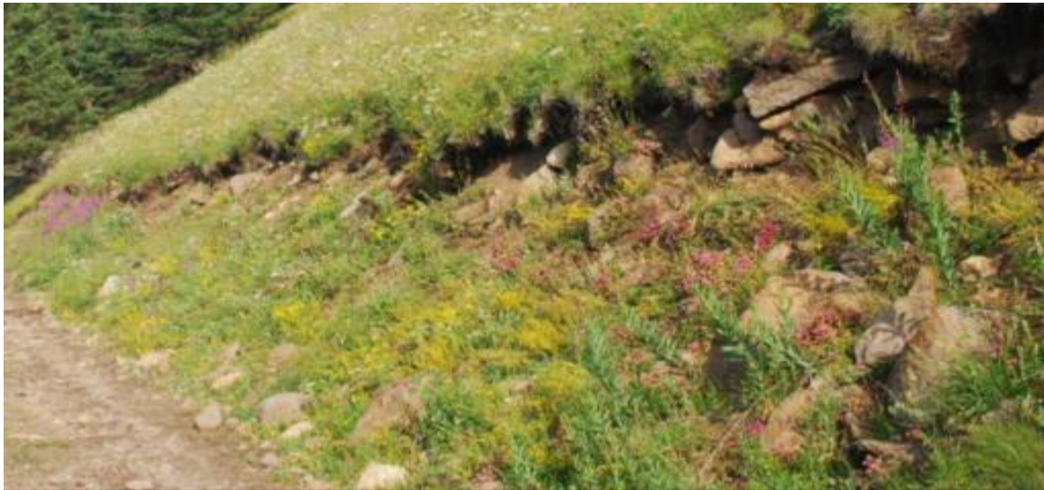
Figure 5.2.4-3. Erosion at steep slope transition.
