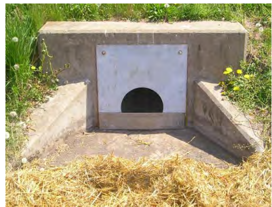
Figure 5.3.13-7. In addition to modifying the basin itself, the outflow structure can be modified to retain volume. A simple weir plate at an existing headwall is often a cost-effective outlet modification. This basin was modified to retain a 4-inch water depth below the weir.
