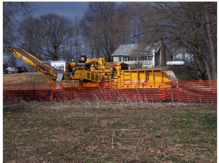
Figure 6-4. Unnecessary material storage and equipment movement can compact soils, resulting in more runoff after construction. Clearly limiting vehicle access to unpaved areas can improve soil conditions adjacent to roadways.
