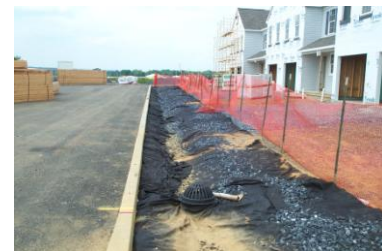
Figure 5.3.1-16. Extending the geotextile over the stone bed during construction of this pervious concrete sidewalk prevents sediment from entering the bed. In this example, the stone bed is wider than the sidewalk. It is designed to manage street runoff (from left) after treatment through a vegetated swale. Runoff sheet flows into the swale over the curb after construction of the final pavement course.
