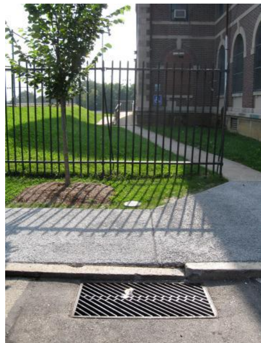
Figure 5.3.3-7. If a catch basin is used to collect street runoff into a tree trench, the inlet must include a sump and a water quality insert to control sediment. This tree trench is built with a porous pavement sidewalk. (Also see Figures 5.3.11a and b.)
