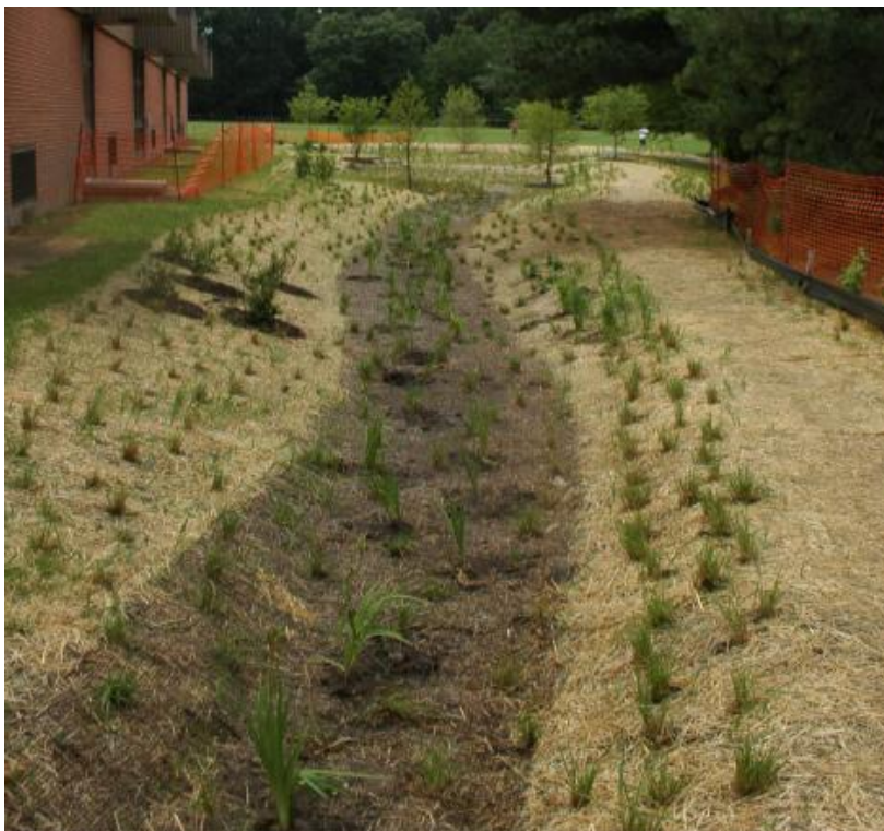
Figure 5.3.5-12. This vegetated swale is stabilized with a temporary turf reinforcement mat until vegetation is established. Careful erosion control is maintained through erosion control materials on the other portions of the site.
