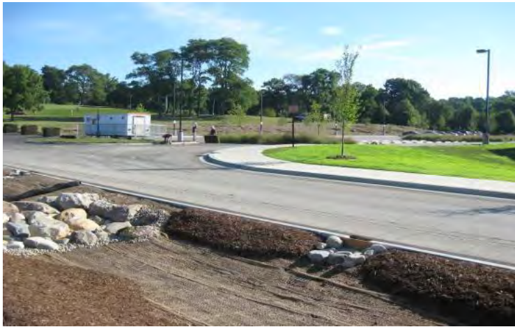
Figure 5.3.4-23. A curb cut is closed to prevent sediment-laden water from entering the bioretention area until site stabilization occurs.
