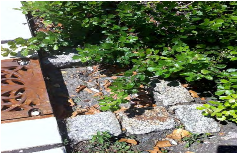
Figure 5.3.4-16. A cobble splash block prevents the movement of sediment into the bioretention area and also allows for routine cleaning and maintenance.
