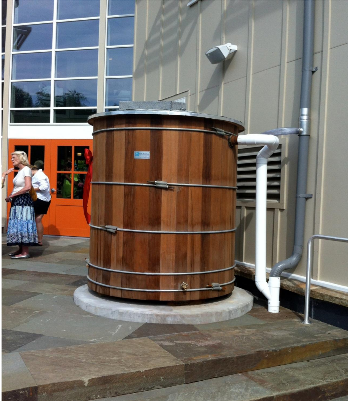
Figure 5.3.9-5. This wooden cistern captures roof runoff at a research facility. The water is used for both toilet flushing and research needs. The captured runoff was more suitable and required less treatment for research use than the available potable water supply.
