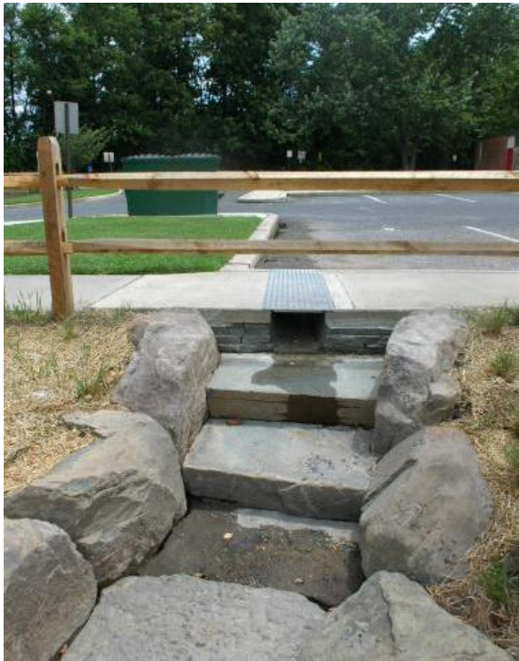
Figure 5.3.5-8. A series of splash blocks prevents erosion on the side of this vegetated swale as runoff enters from a parking lot via a trench drain.
