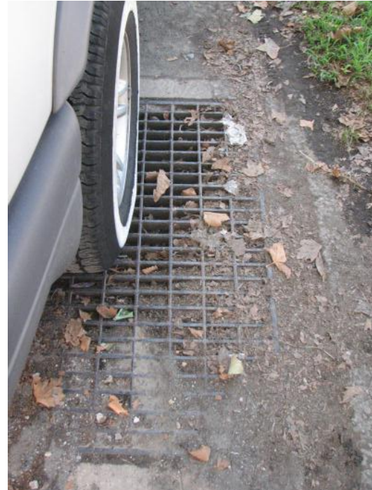
Figure 5.3.3-9. Lack of inlet maintenance can prevent water from entering an urban tree trench.
