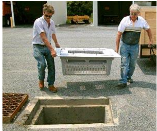
Figure 5.3.2-11. Water quality inserts can be used to reduce sediment and prevent trash from entering a stormwater infiltration bed. Water quality inserts require regular maintenance. ( http://www.gaelwolf2.com/dnrec/trib_times_2004_4_catch_basin_inserts.htm , Aug. 24, 2012)
