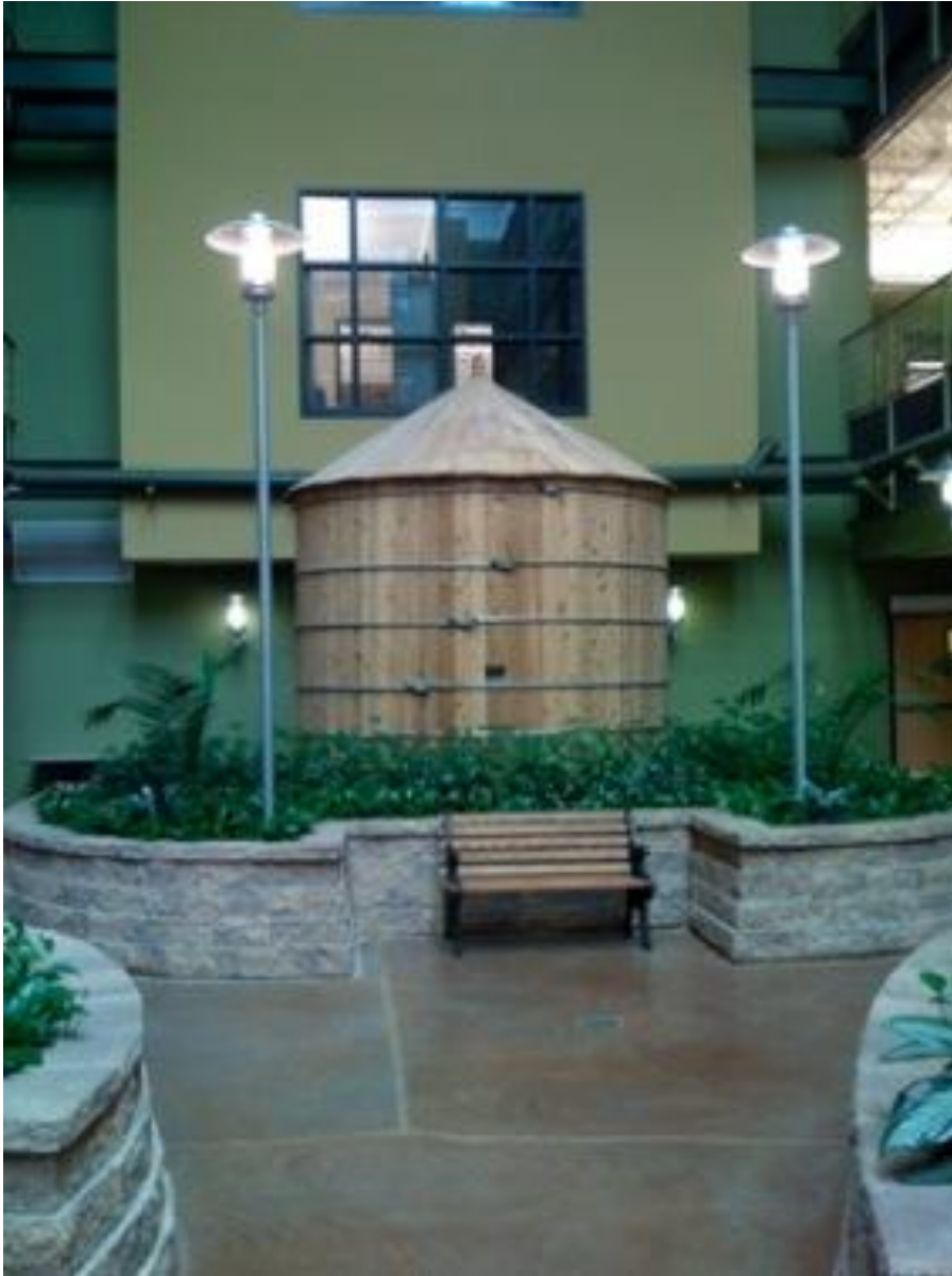
Figure 5.3.9-6. This cistern is located indoors. Roof runoff is captured for toilet flushing within the building.
