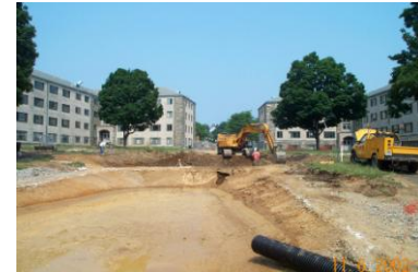
Figure 5.3.1-12. The stormwater bed beneath this pervious concrete plaza was used as a temporary sediment basin (with basin bottom at least 2 feet above final stormwater bed bottom elevation) during construction of the site. After the surrounding site work was completed, the sediment was removed and the bed excavated to its final depth. The stormwater bed and overlying pervious pavement were then installed.
