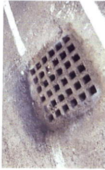
Grease evidence at storm grate. Grease was discharged into stream. Enforcement action was taken.
